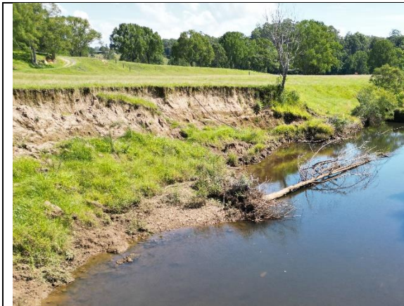
Plate 7 Section E – Bank slumping with gravel deposit at toe
