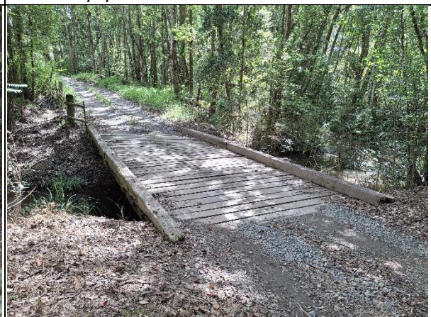
Photo 6: Wooden Bridge which will need bridge strengthening works Date: 20/3/2025
