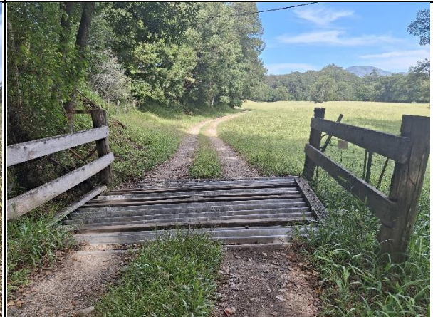
Photo 4: Cattlegrid which will need strengthening with a steel plate Date: 20/3/2025
