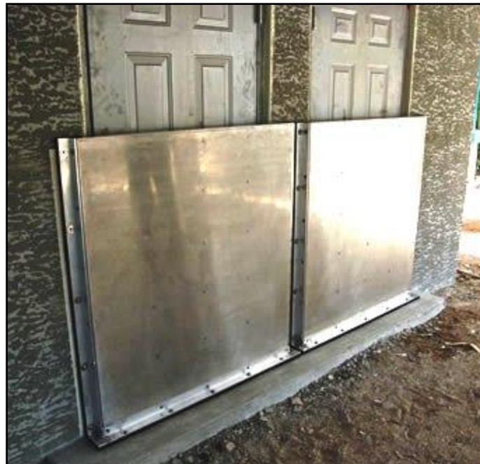
Photo 2: Dry proofing on doors of residential property
