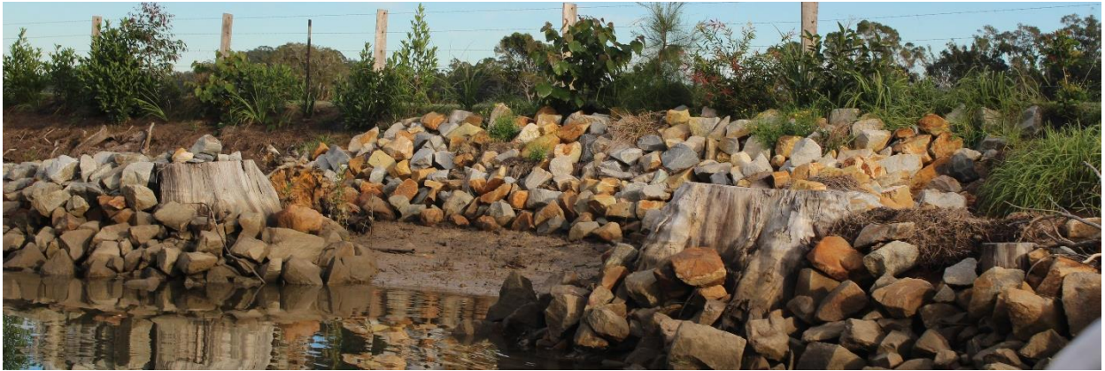
Figure 29. Rock fillet bank stabilisation works recently implemented in Kalang River lower estuary
