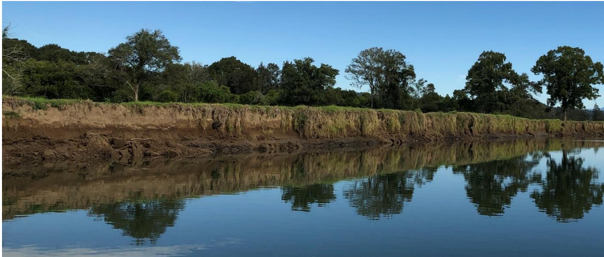
Figure 25. Major bank erosion within the Bellinger River upper estuary
