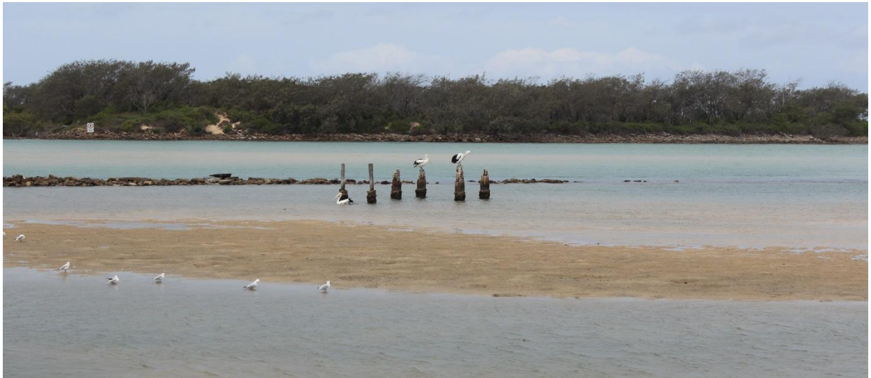
Figure 27. A section of rock training walls at the Bellinger-Kalang River estuary entrance
