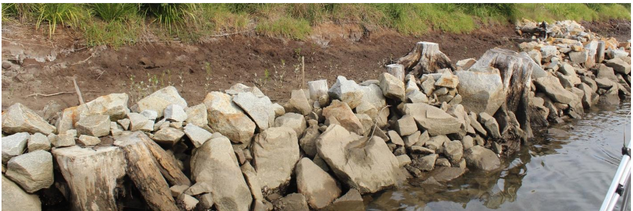
Figure 30. Rock fillet bank stabilisation works recently implemented in Kalang River lower estuary
