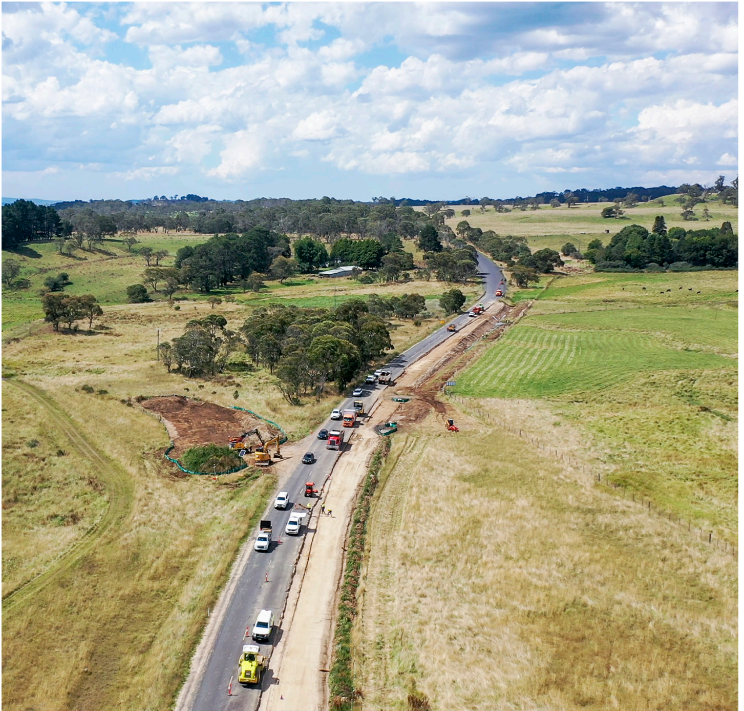
Construction work between rabbit eradication fence to Ebor tip, east of Ebor
