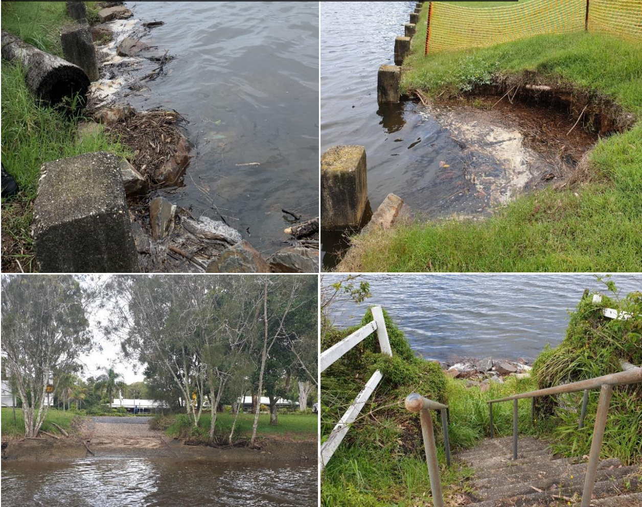
Figure 10 Damage to infrastructure at Mylestom Reserve foreshore.
