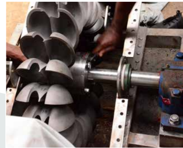
Talise hydro, Vanuatu - Pelena Pelton turbine
