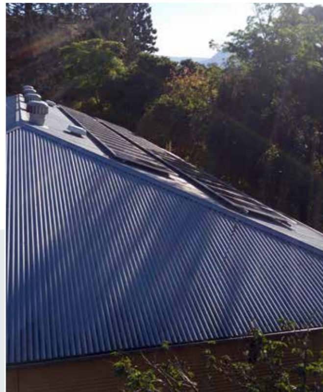
Roof top Solar PV, Bellinghen Shire
